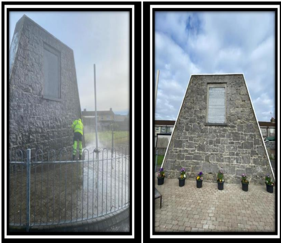
REFURBISHED 'TUAM MARTYRS MEMORIAL' AT THE SITE OF THE FORMER WORKHOUSE IN TUAM, CARRIED OUT BY CES TEAM. NOTE THE WRITING ON THE PLAQUE HAS ALSO BEEN REDONE.
